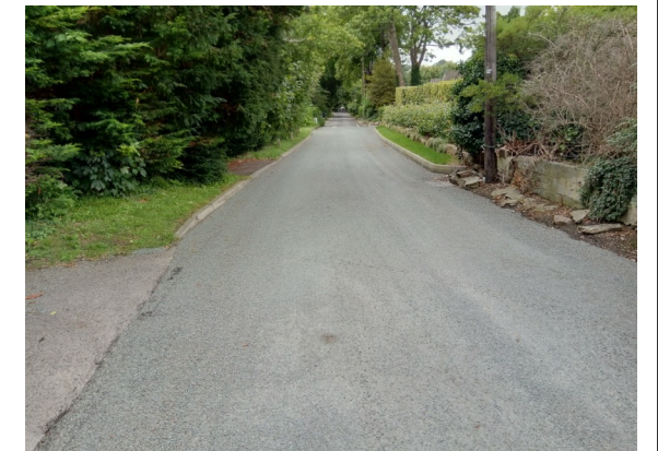
Surface dressing in Welcomes Road by Allfreys using 6mm granite chips is holding up well
